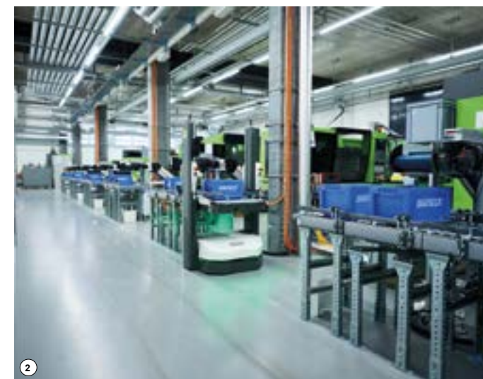
① The flow racks comprise 60 channels on 4 levels. The Open Shuttle transfers the molded parts automatically to the allocated channel, then removes empty containers and brings them to the injection molding machines.
